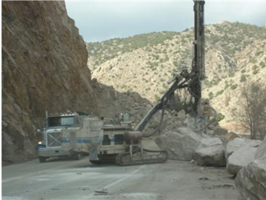
Figure 12-6. Highway 50 Rockslide Cleanup
