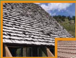
Figure 8: (above) Wood shingle roofs are highly flammable and not recommended. Photo: CSFS
